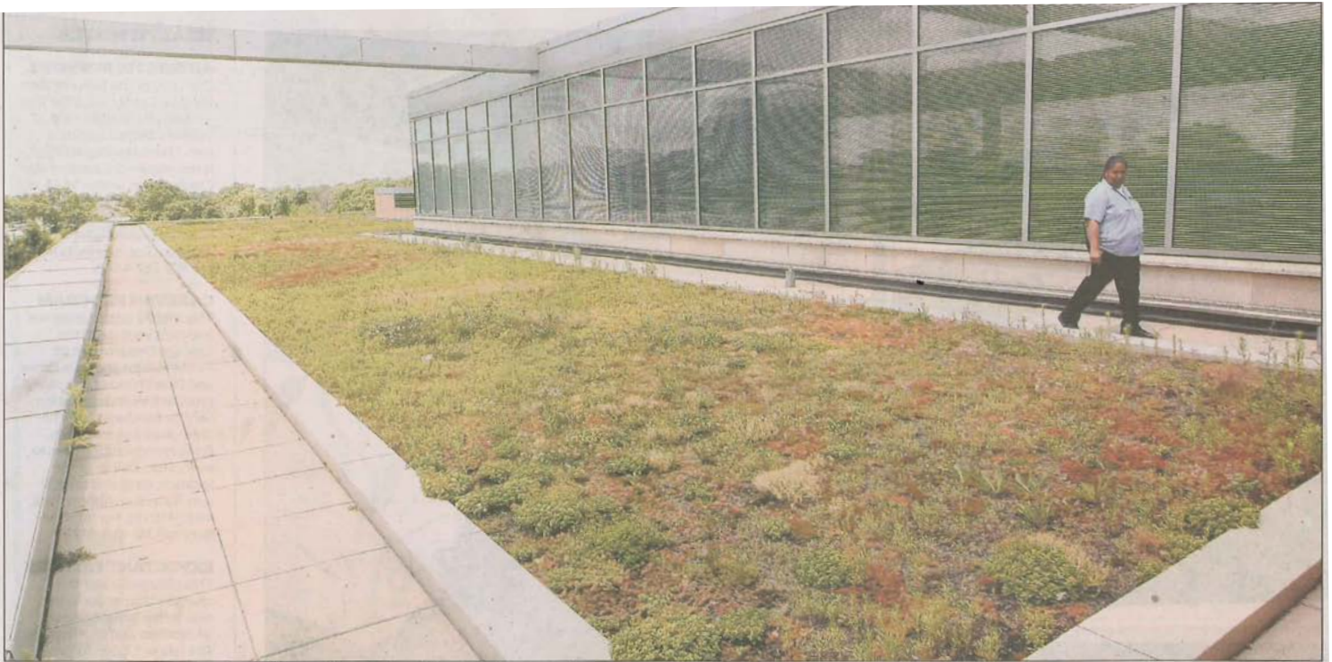
Custodian Joyce Hicknbottom checks the roof-top garden Friday at Tarkington School of Excellence, the Chicago Public Schools' first so-called green building. PHIL VELASQUEZ/TRIBUNE PHOTO
